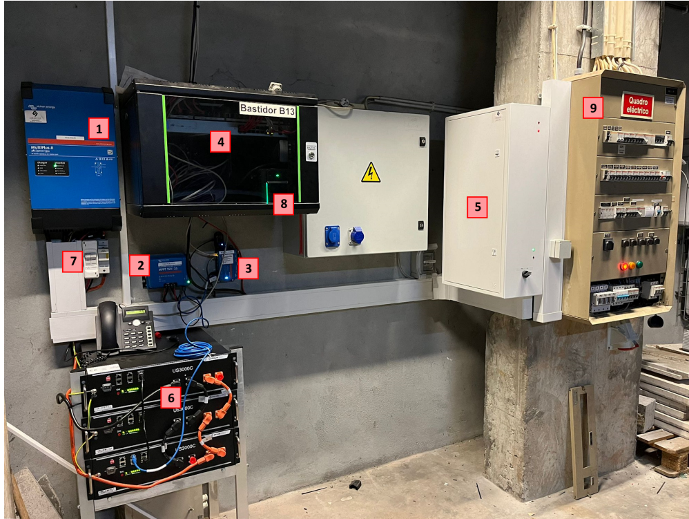
Figure 3.6: Photo of the On-Site Installation.
