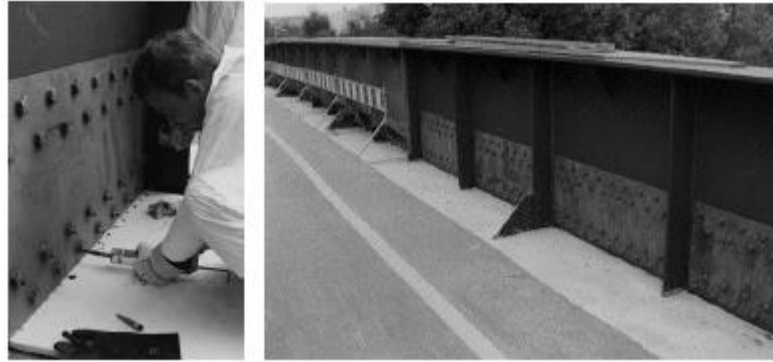
Figure 2.21. Strengthening operations of the web in the main girder using injection bolts [20].
