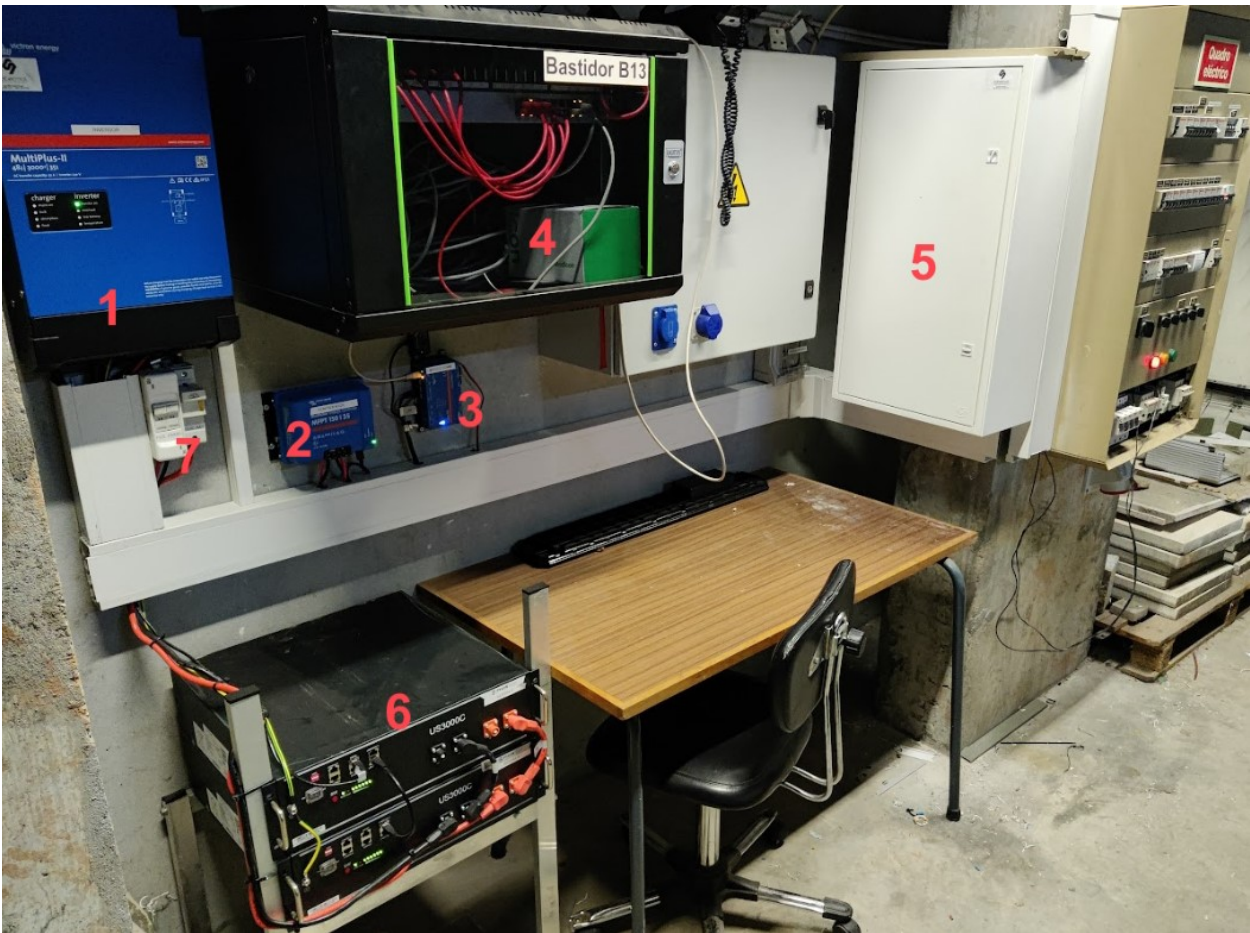
Figure 3.1: Photo of the On-Site Installation.
