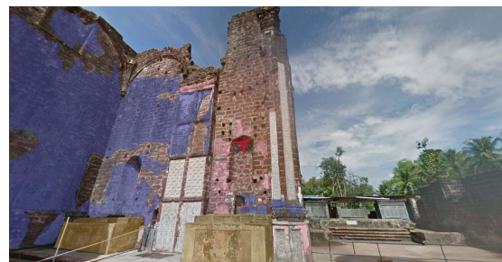
Figure 89: Diagnosis on the remains on the left of the transept of the Church on Base Fig.88.
