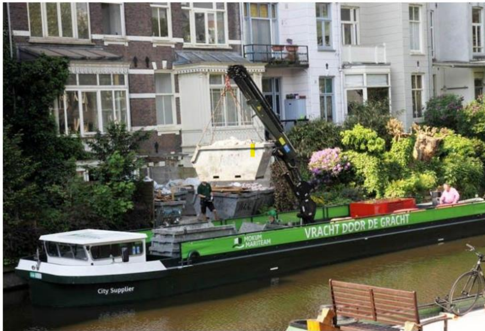
Figure 20 - The Mokuem Mariteam Barge Loading Construction Waste with Its Own Crane (Zacharopoulos, El, Supervisor, & Gonzalez-Aregall, 2020).
