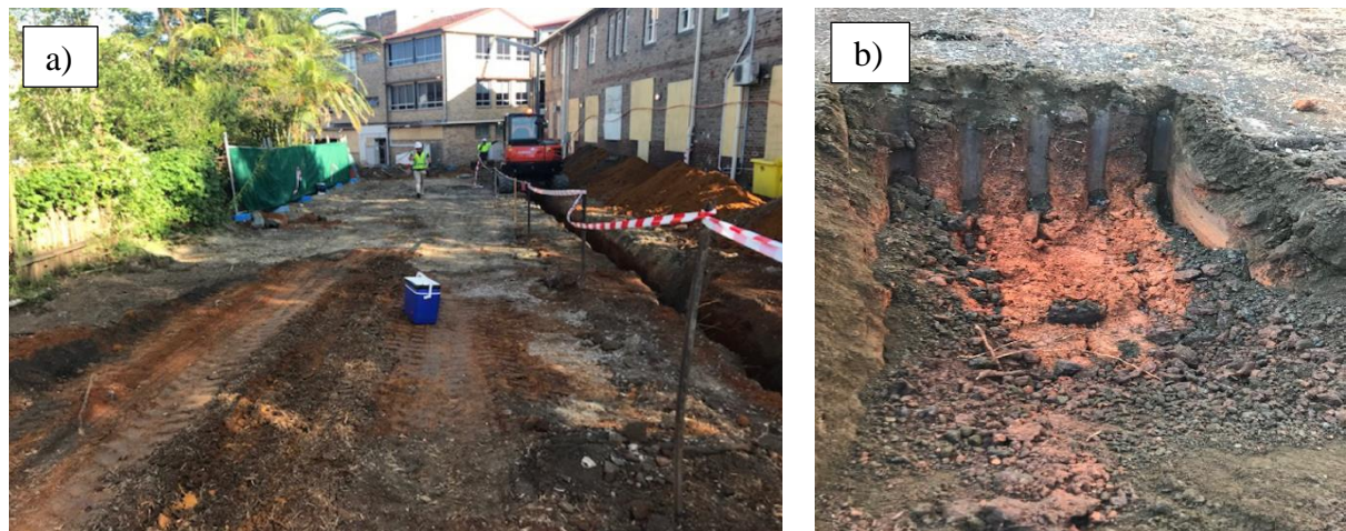
Figure 3.8 North Sydney Council (a) View of site conditions. (b) View of sub-surface conditions. (EI Australia, 2020)
