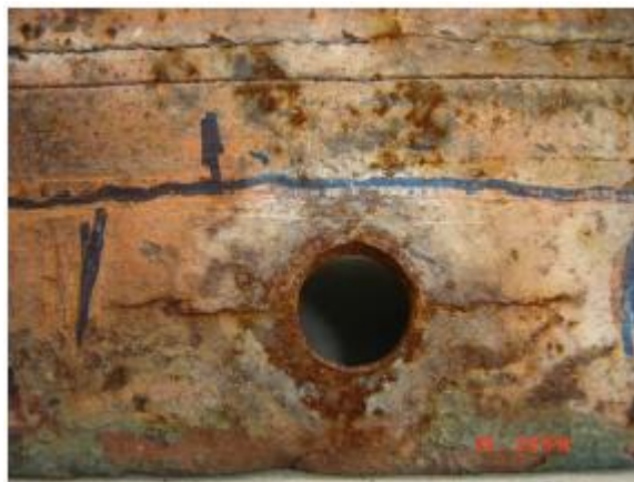
Figure 1.1 – Fatigue crack growing from a rivet hole (Jorge et al , 2006)
