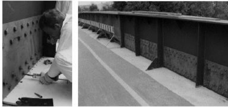
Figure 3.2 – Strengthening operations of the web in the main girder using injection bolts (Gresnigt et al 2000)
