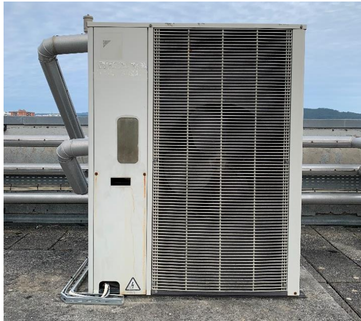
Figura 3.12 Chiller Daikin EUWA5GW1.
