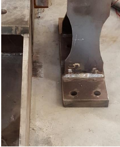
Fig. 5.184 – Displacement of the column base
