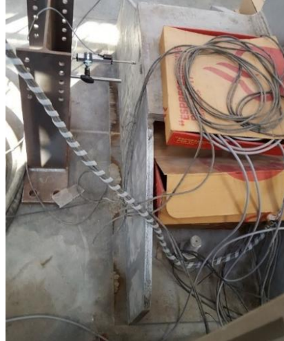
Fig. 5.185 – Displacement of the steel braced
