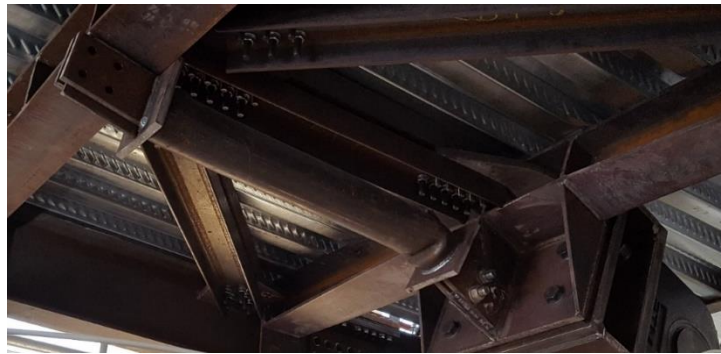
Fig. 5.182 - Structural elements after damage
