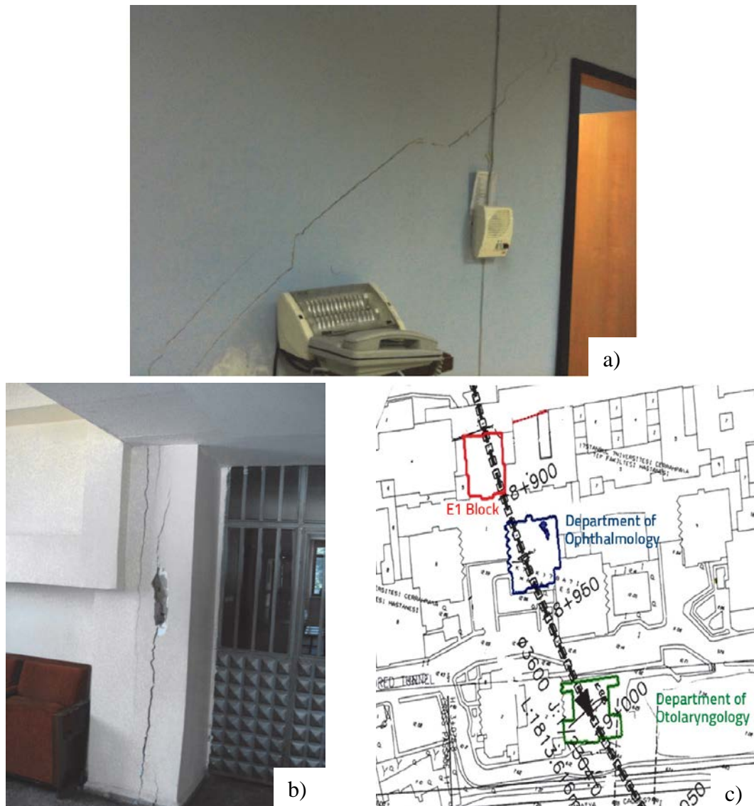
Figure 3- Pictures obtained from the buildings in the Medical Faculty: a) diagonal cracks formed in a wall of the basement floor due to bending; b) shear and compression crack a column of one of the buildings; c) route of the tunnel and location of the buildings highlighted from the Medical Faculty (Yildizlar et al.,2014)
