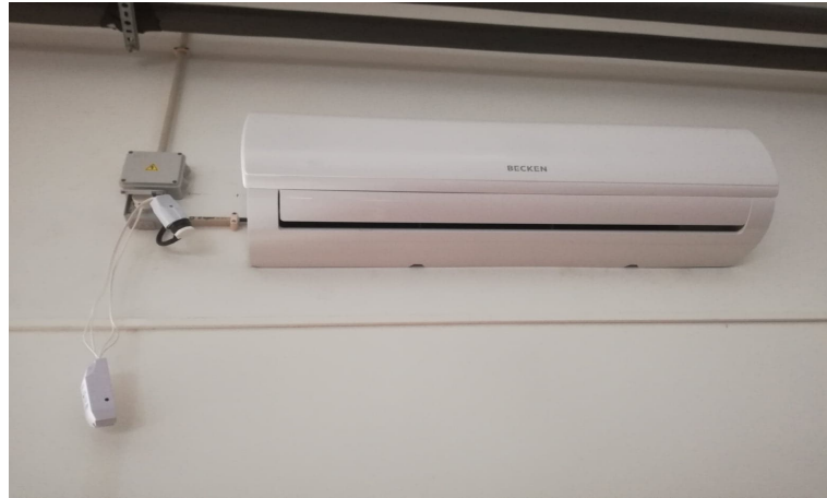
Figure 4.1: The AC system to measure the electric power consumption.
