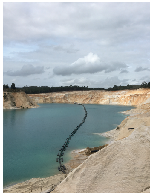
Figure 3.3. Dredger working inside the Via-Vai quarry and pipeline transporting sand for processing.
