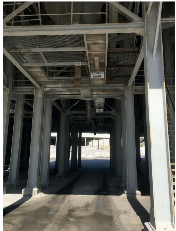
Figure 3.18. Underneath storage silos with outlets labelled with the product.
