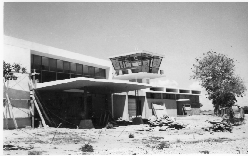
Figure 10. João José Tinoco and Maria Carlota Quintanilha. Pemba Airport under construction. Mozambique, 1959–1961 (photograph, circa 1960). (Credits: Author’s archive).
