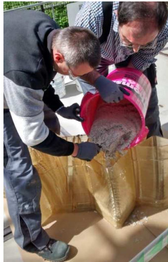
Figure 2-24 – Engineers at the 3D Print Canal House pour concrete in 3D printed molds[62].
