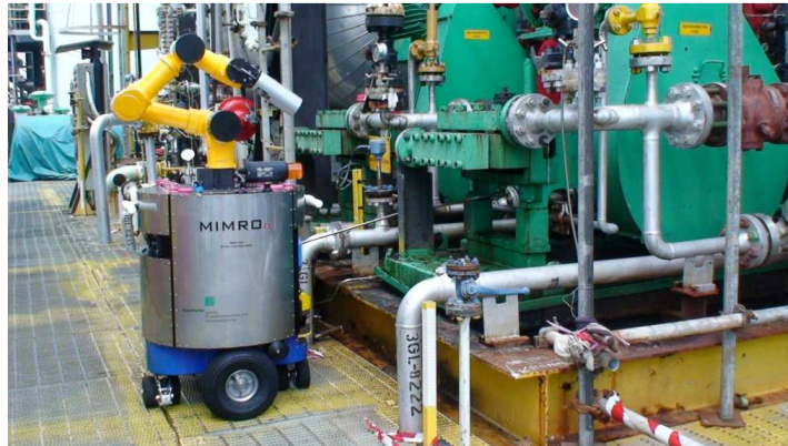
Figure 2-5 - Fraunhofer MIMROex robot inspecting a process plant during field test on the topside of a platform[28].
