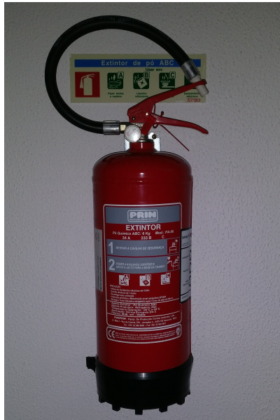
(a) Fire extinguisher
