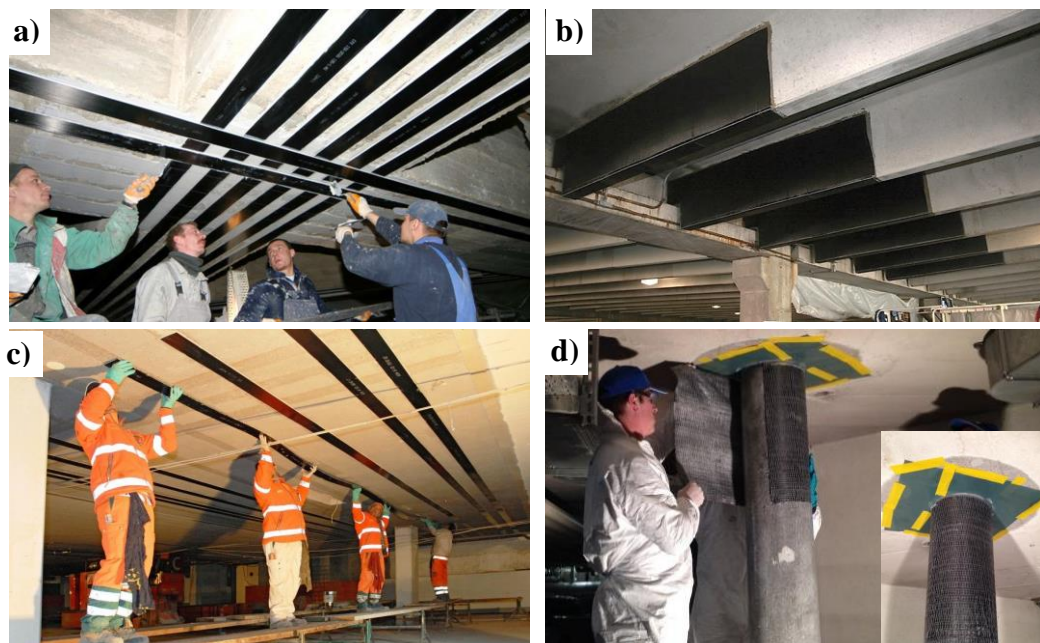
Figure 1.6 – (a) flexural strengthening of RC beams with CFRP laminates [18]; (b) partial shear strengthening of RC beams with CFRP sheets [19]; (c) flexural strengthening of slabs with CFRP laminates [20]; (d) strengthening to axial stress and confinement of columns with CFRP sheets [21]
