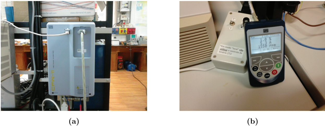
Fig. C.5: VSD used for primary machine control: (a) VSD; (b) VSD's remote controller
