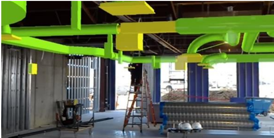
Figure 2.15 – “Project Monitoring” App by Trimble being used to aid in the construction of a system of pipes
