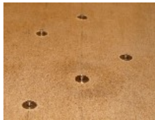
Figure A2-10: Detail of the Irwin probes surface-mounted on one of the piles.
