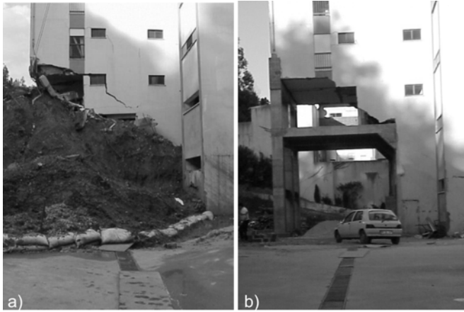
Figure 3 - Accumulation of soils against the building at the foot of the earth flow, which destroyed two floors, leaving the remaining twelve floors suspended. a) After the failure; b) One year later, after repairing the affected concrete structure.
