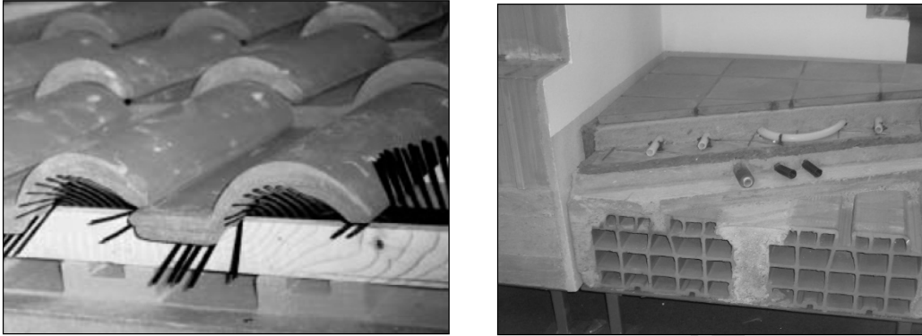
Fig.1 Constructive details: ventilated roof and floor with under-floor heating design and practice
