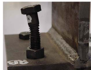
(b) Detail of an unbroken bolt after failure of the connection.
