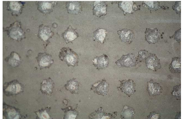
Fig. 4. Substrate surface partially chipped.
