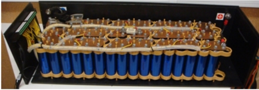
Figure 3.2: Lithium-Ion battery pack acquired to the company Autosil S.A. (72V, 3kWh, 24 modules in series with 4 parallel cells each - 4P24S).
