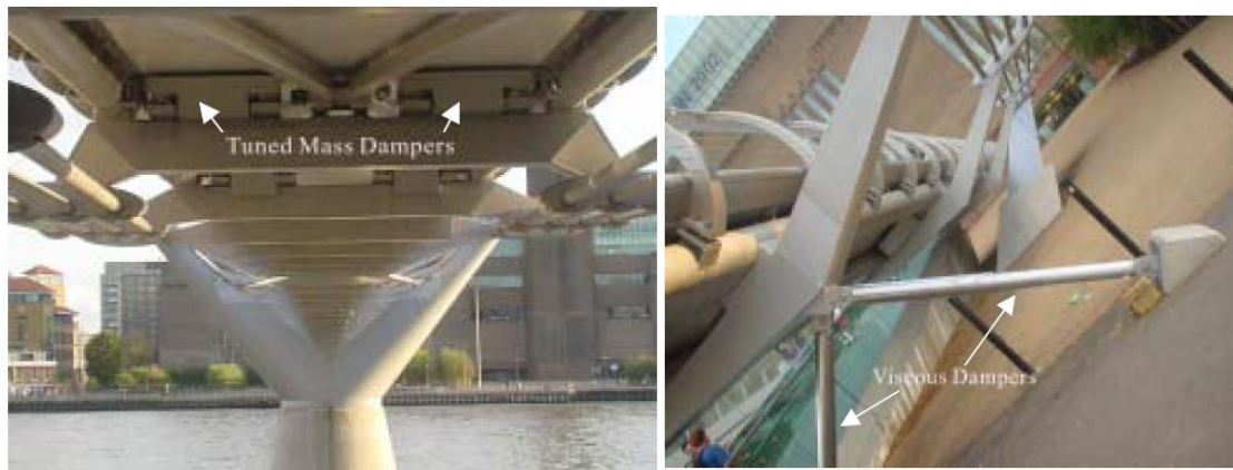
Figure 2.4- Tuner mass damper and viscous dampers installed in the London Millennium Bridge (Mualla & Nielsen n.d.)
