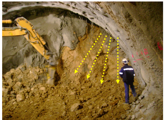
Fig. 5. View of an instability with a distorted light umbrella in Zone 2 (section 70).
