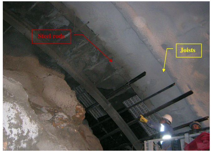
Fig. 4. Detail of the support with an umbrella of steel rods 4 m in length and packed with light beams.
