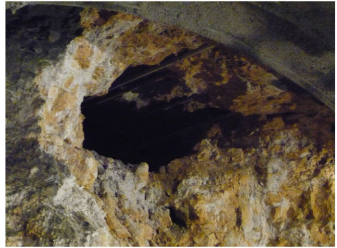
Fig. 6. View of a cavity of approximately 20 m 3 affecting sections 206 to 210.
