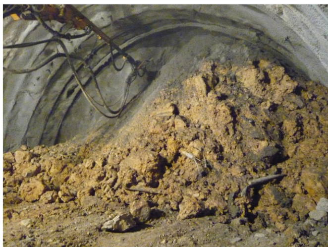
Fig. 7. View of the large instability affecting section 302, obliging to stop the work in the tunnel.
