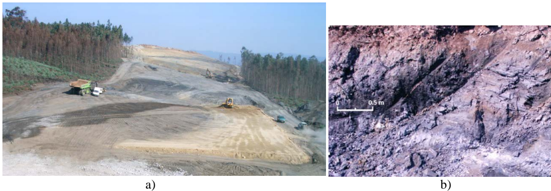
Fig. 2 a) View of construction site with black shale mixed with brown schist; b) detail of the black shale.
