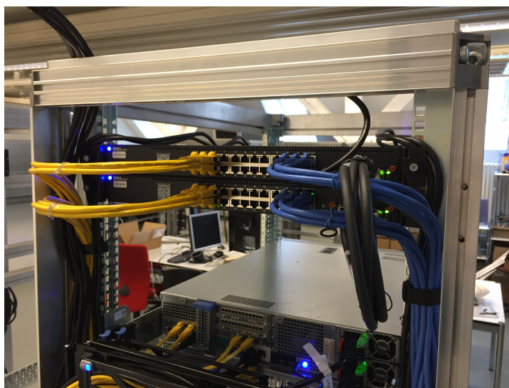
Figure 3.2: Cloud Computing Testbed Switches
