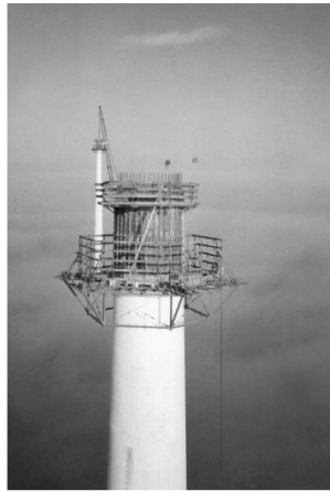
a. Construction of a tower for an Enercon E-66 with site-mixed concrete
