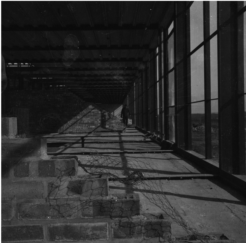
Photograph showing the interior of Hunstanton Secondary Modern School, Norfolk, during construction [c 1953]
