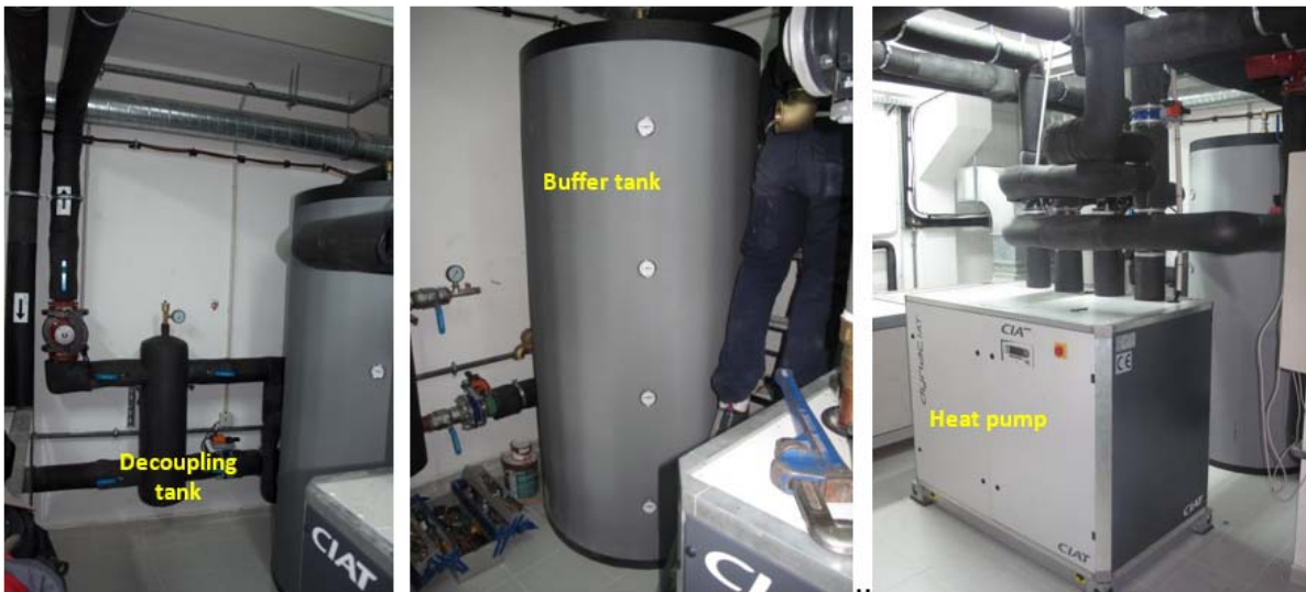
Figure 3.8: Pictures of the HP and associated equipment machinery room.
