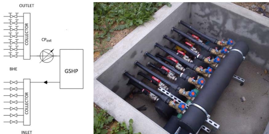
Figure 3.10: The seven pair of tubes connected to the collectors.
