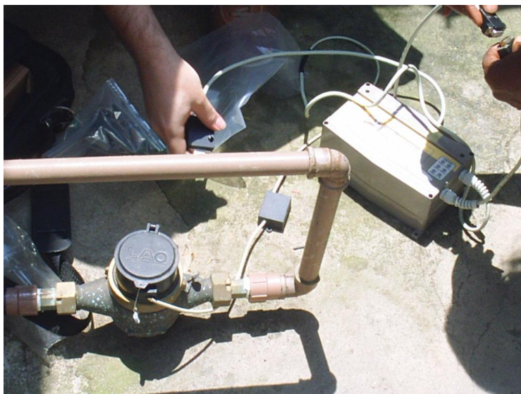
Figure 5.6: Water-meter and data-logger used for water consumption investigation in Brazil
