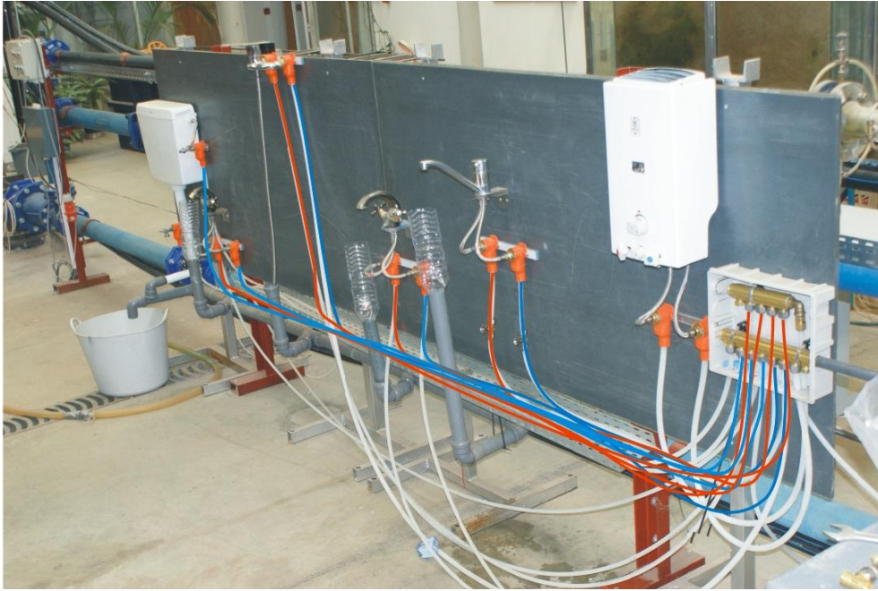
Figure 3.20: Unequal pipe length was set up at the experimental facility.
