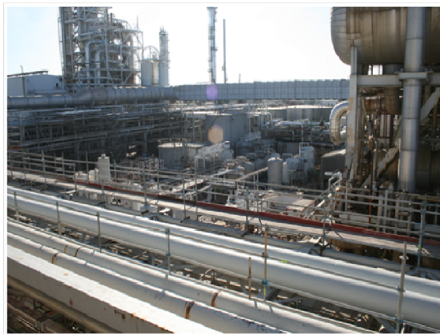
Fig. 5.1 A Typical Part of an Oil Refinery
