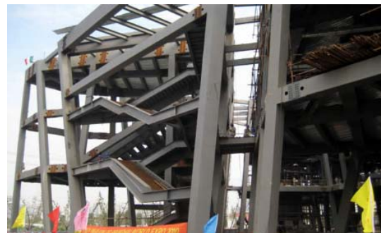
(b) Members with polygonal centroidal axis (stairs) – Italy pavilion, World Expo 2010 – Shanghai
