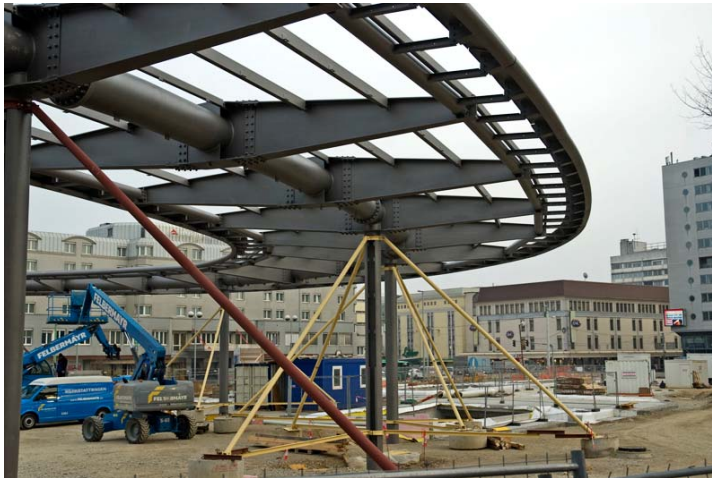
Figure 1.8 Construction site in front of the Central Station, Europaplatz, Graz, Austria (Nahverkehrs-drehscheibe Graz-Hauptbahnhof, 02-02-2012 [online])
