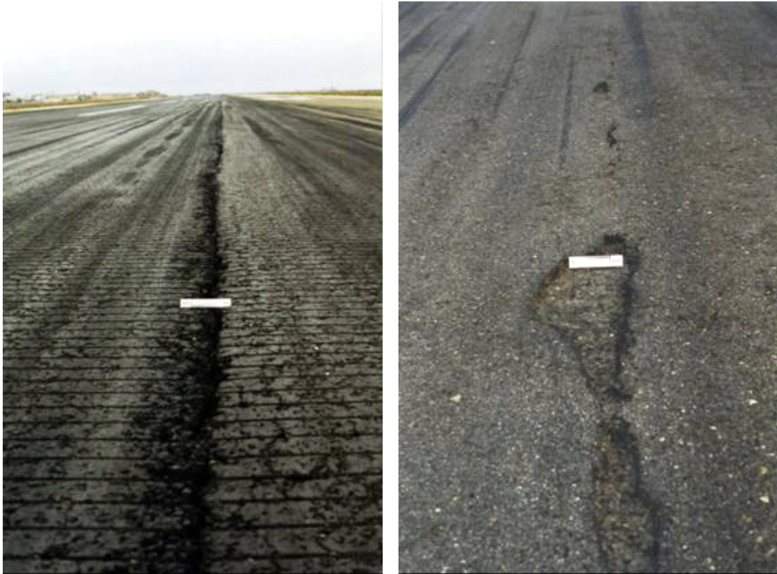
Figure 7.2 – Pavement surface condition: longitudinal joint (left) and pothole (right)
