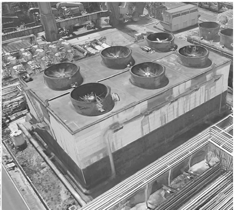
73 - East Thermoelectric cooling building (Northeast view)
