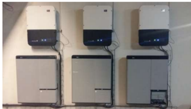
Figure 3.1: Energy Storage System [23]
