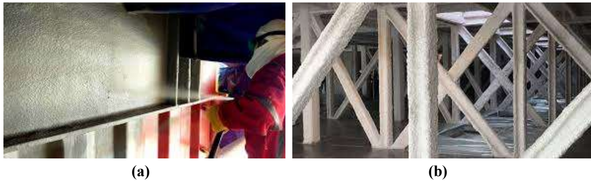
Figure 2.4 – Passive fire protection sprayed mortar under application procedure (a) and after the application in steel structures (b) (from Ref. [55-56], respectively).
