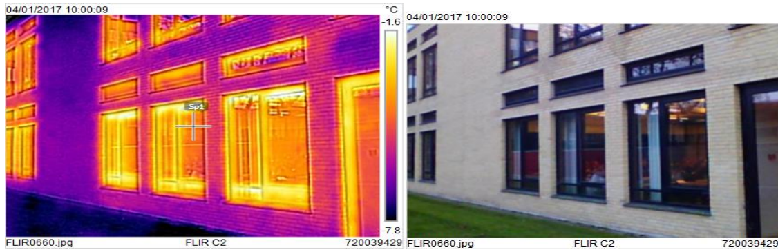
Figure 34 shows insufficient insulation on the outer wall and high heat loss
