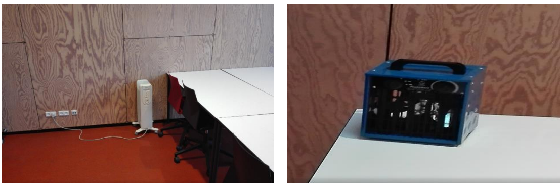
Figure 19 shows the electrical heater used in the building, which indicates that the heat delivered from the central heating system does not deliver as much heat as was estimated.
